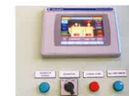
PLC display(panel view) facilitating the monitoring operation condition
