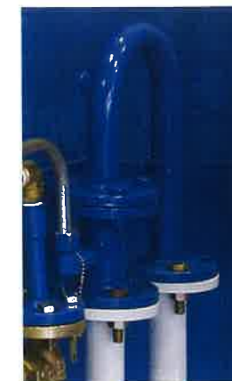
Self-Cleaning strainer in the sludge long
